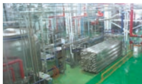
前處理設備 Pre-treatment equipment
